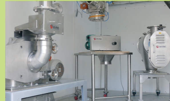
Well equipped test room in Düringen
